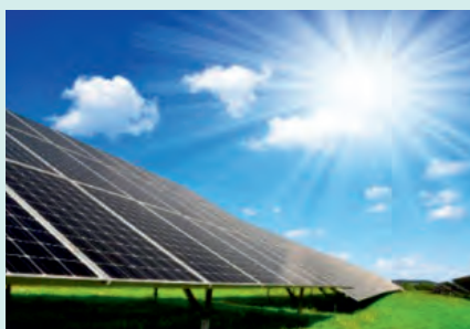
Ground mounted solar
