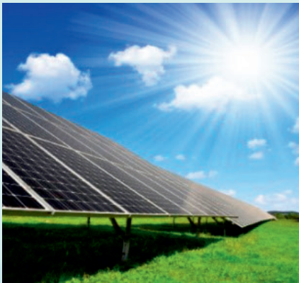
Ground mounted solar
